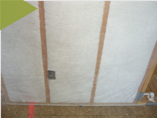
NO AIR GAPS AROUND OUTLETS
